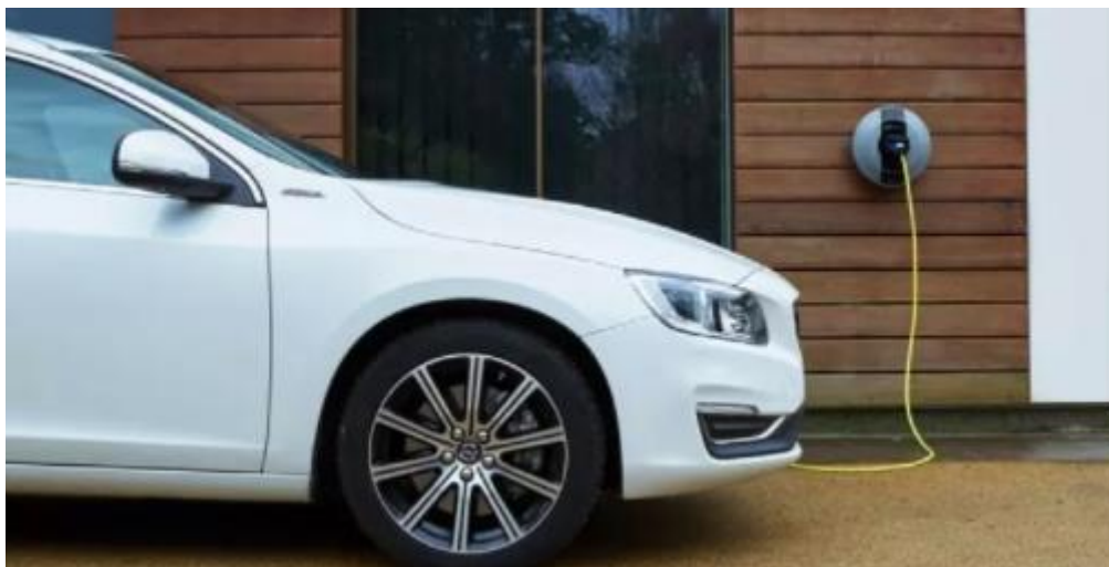
Figure 8. Residential charging point
